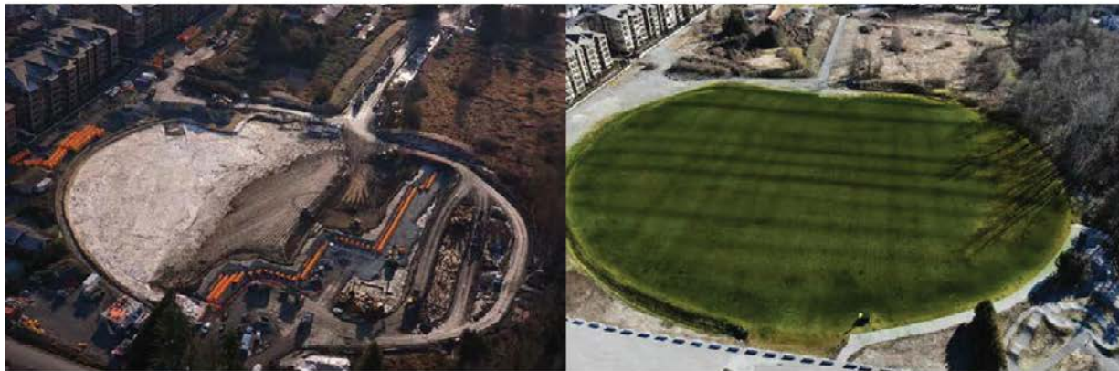
Figure 1: Before and after. Upon completion, this is now one of the largest underground stormwater detention systems in North America.
