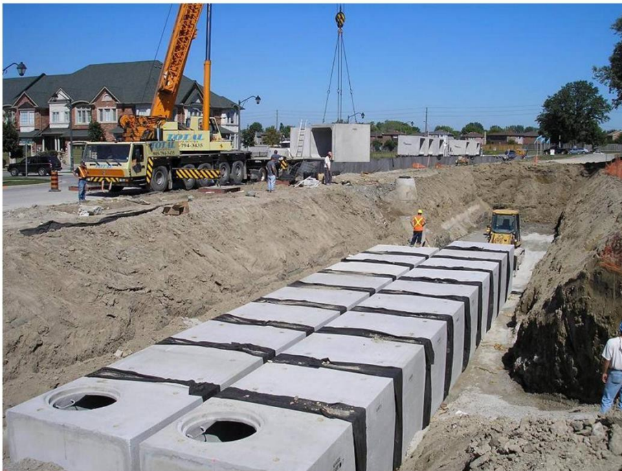
Subsurface Stormwater Storage Facility
