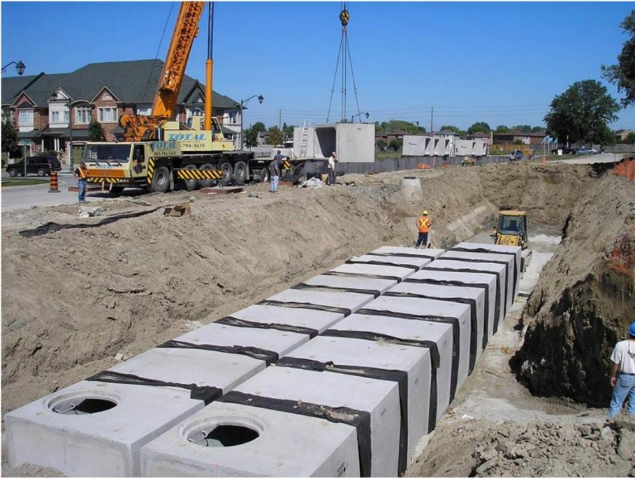
Subsurface Stormwater Storage Facility
