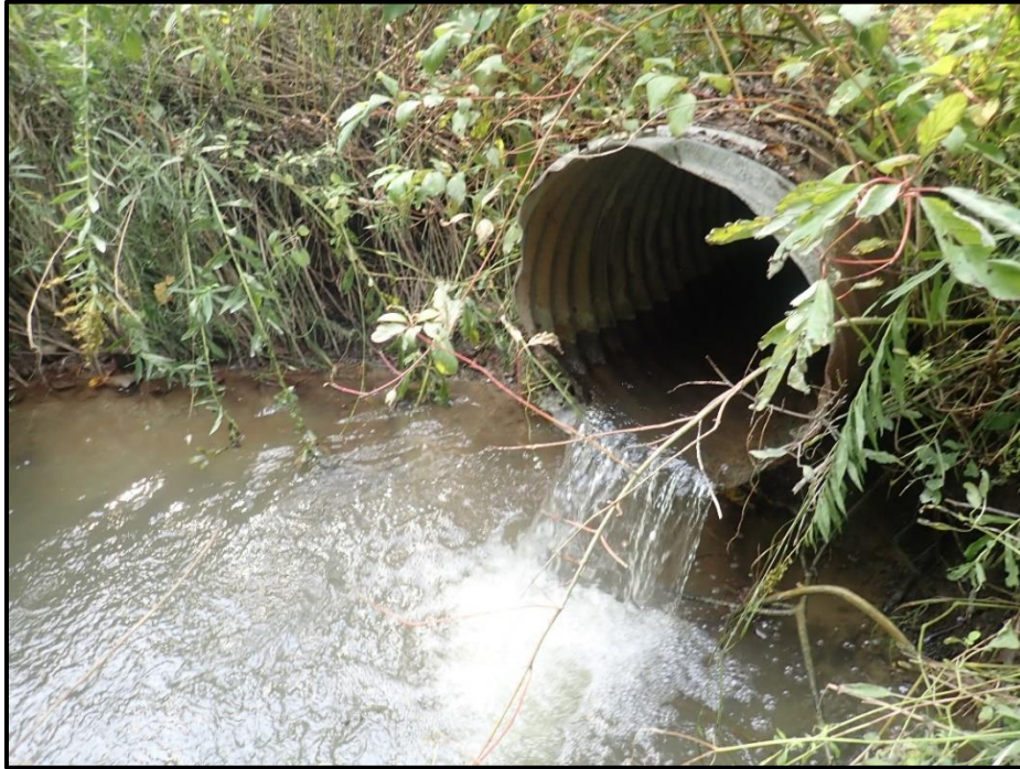
Photograph 5. Tannery Creek West Tributary – Perched Culvert (September 16, 2020)
