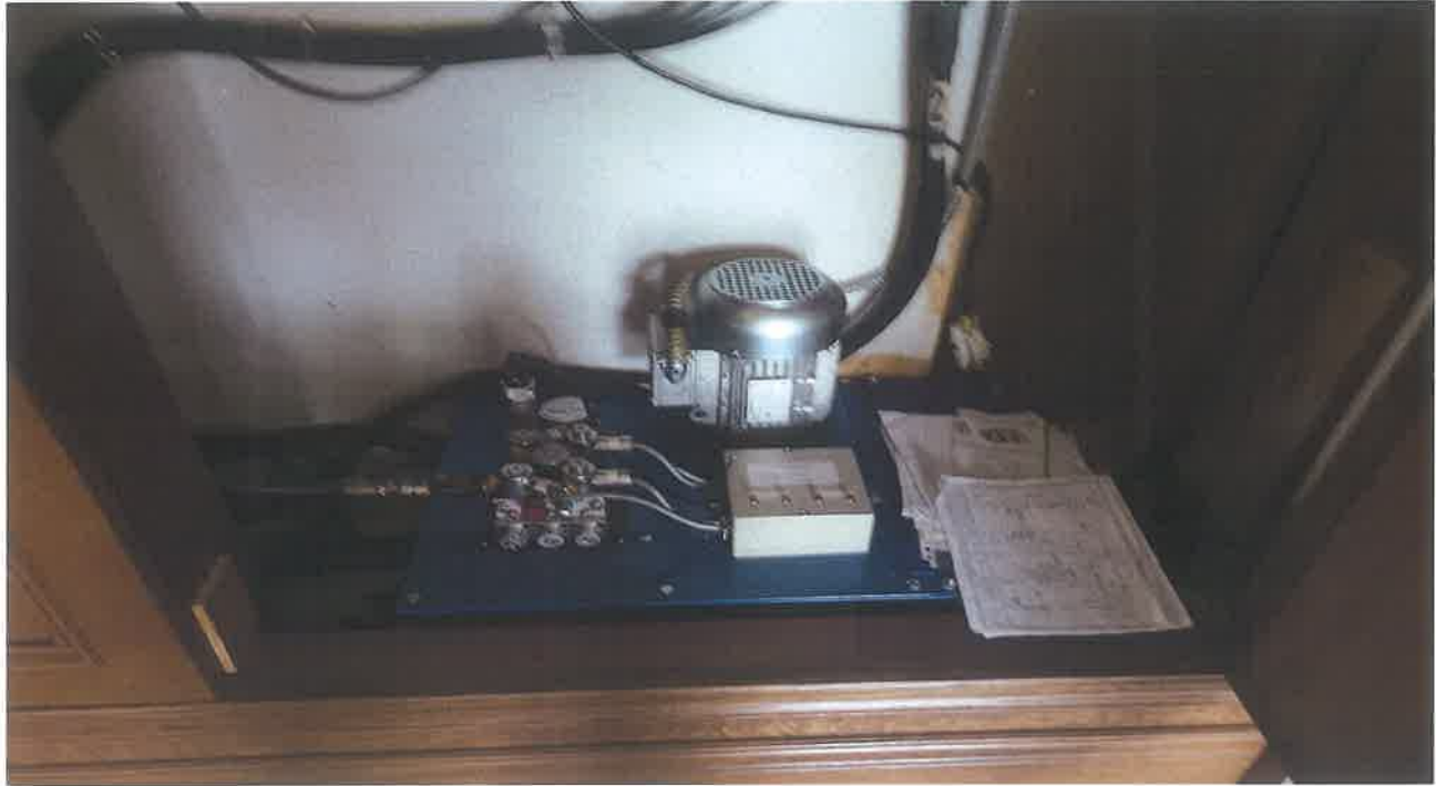
Generator for elevator in West Subject Site Residence
