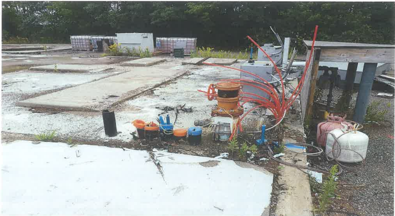
Utility area of former skating rink at central portion of Subject Site (looking East)
