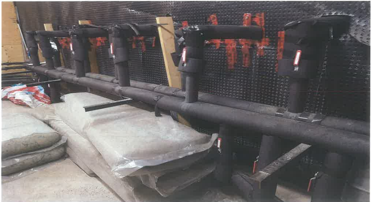
Geothermal intake at West Subject Site Residence
