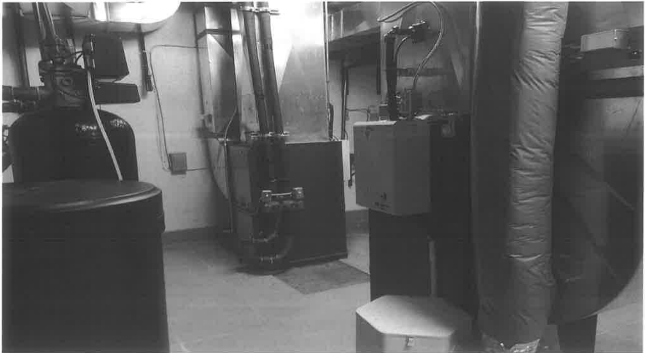
Furnace and Water Tanks in West Subject Site Residence (looking North)
