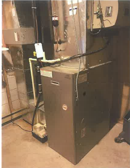
Furnace in basement of Residence at East portion of Subject Site
