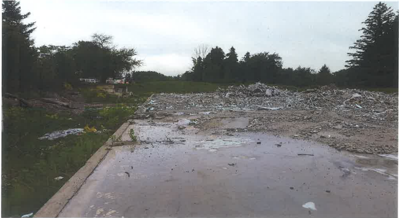
Demolition of former skating rink at central portion of Subject Site (looking North)
