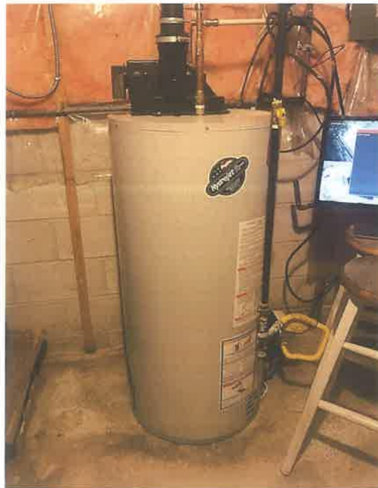
Water tank in basement of Residence at East portion of Subject Site
