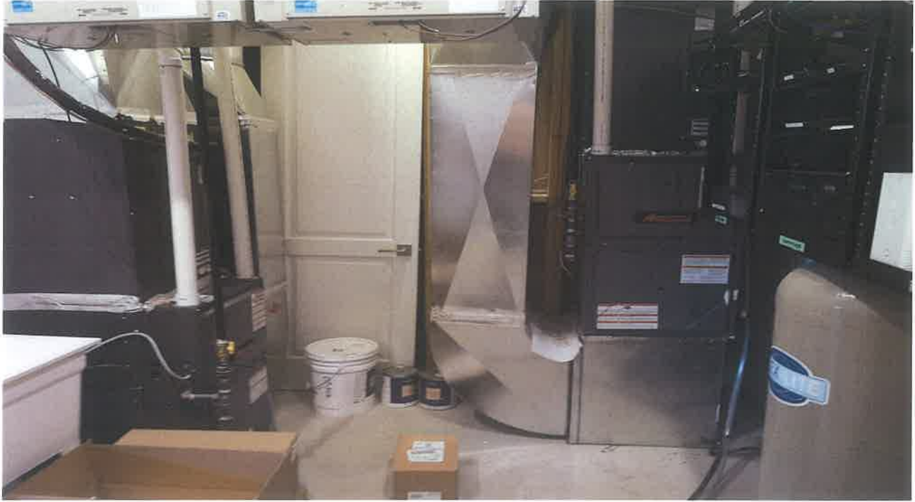
Utility room of Sales Office near East boundary of Subject Site
