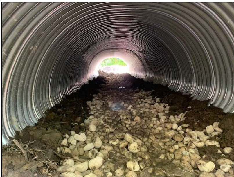
Example of An Enlarged Culvert Designed to Facilitate Wildlife Passage with Terrestrial Clay Benches - City of Burlington
