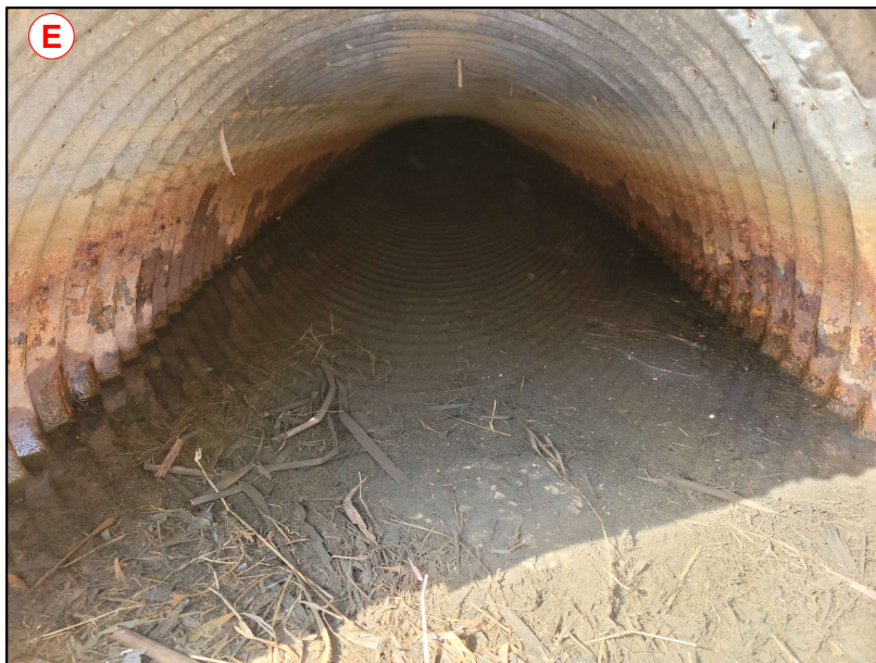
CSP Culvert Beneath Henderson Drive. Note Signs of Corrosion and Loss of Capacity Due to Sediment Accumulation
