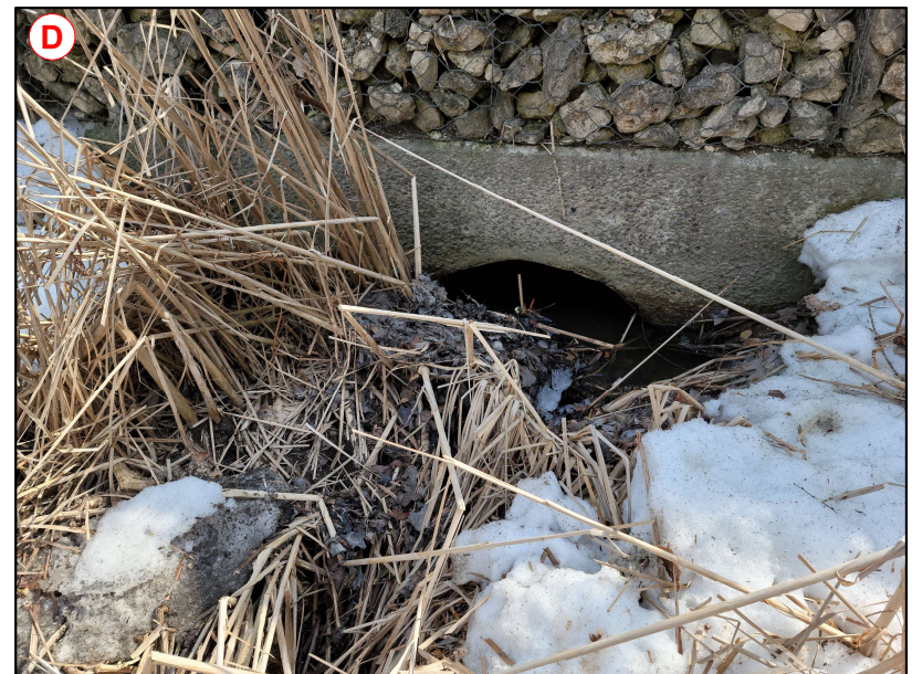
Existing Culvert Outlet. Note Significant Loss of Conveyance Capacity Due to Sediment Accumulation
