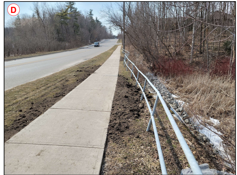
Failing Guard Rail on the North Side of Henderson Drive
