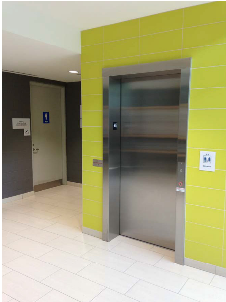
Independent Elevator Access at AFLC
