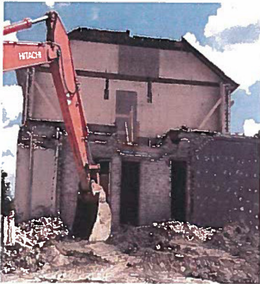
DEMOLIITON IN PROGRESS AT 32 WELLINGTON STREET EAST. DEVELOPER HAS ADEQUATELY UNDERPINNED AND SHORED AS PER THE PERMIT REQUIREMENTS.
