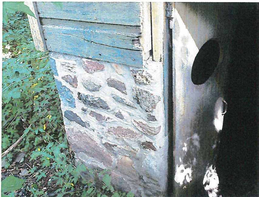
Photo of existing foundation and door, south west corner of the barn.
