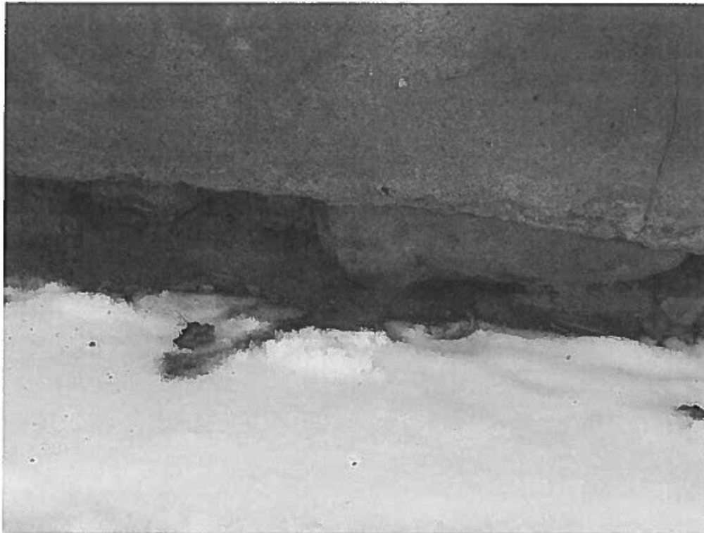
Photo 3. Deterioration of mortar along the west driveway.
