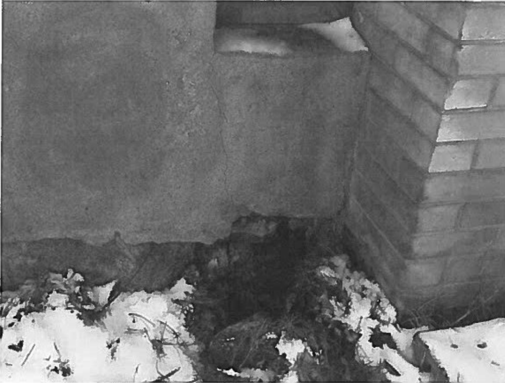
Photo 4. Loose foundation stones along the west side.
