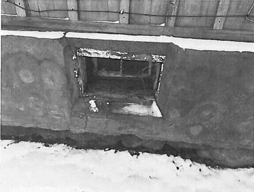
Photo 2. Deterioration of mortar along the west driveway.
