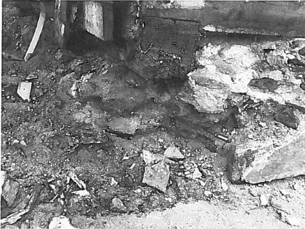
Photo 1. Failed foundation and deteriorated sill beam at north-west corner.
