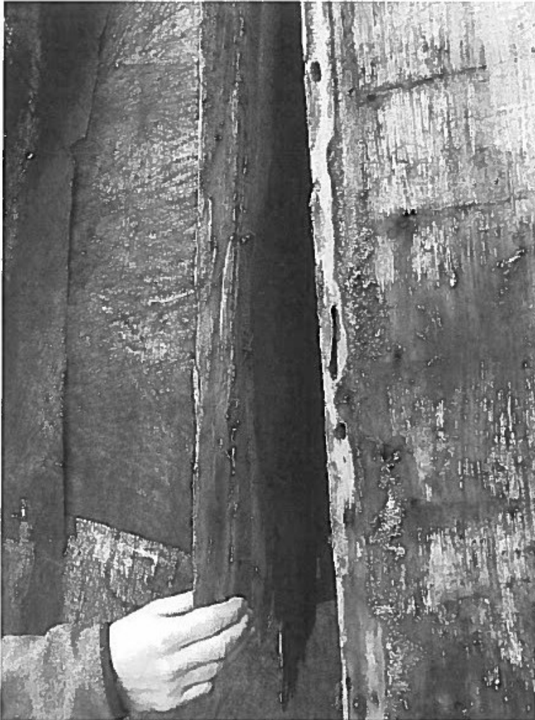
Photo 6. Evidence of carpenter ant activity in the walls above the sill beam (wood shavings and ant galleries).
