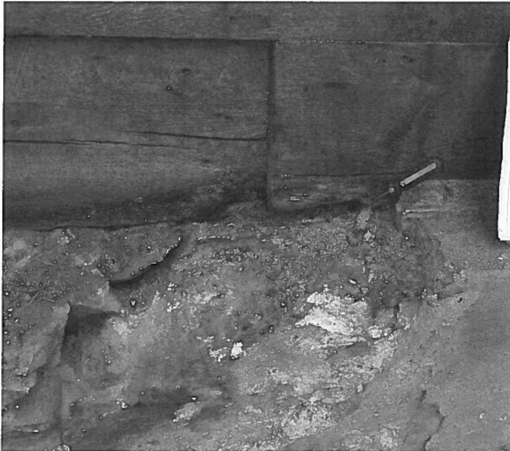
Photo 5. Deteriorated sill beam along the west foundation wall.
