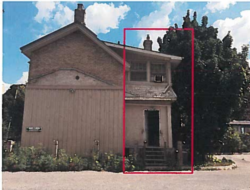
15032 Yonge Street - Rear Elevation (looking east). Addition proposed to be demolished (shown in red outline) is located on the right. The original wing proposed to be preserved, is to the left.
