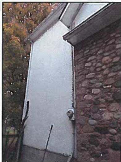
Figure 9: Right and Below: West wall showing edge of two storey north addition and recladding plus a change in the window of west roof gable, 2016
