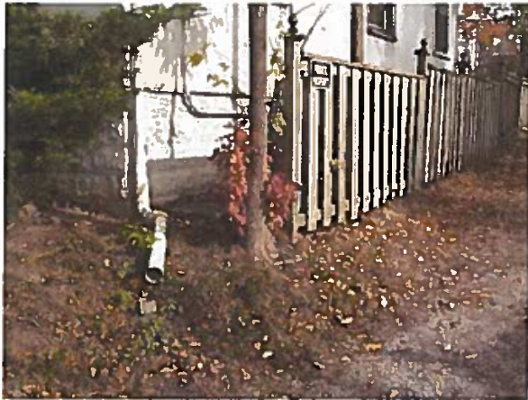
Plate 7: Driveway of 57 Temperance showing driveway cut below surrounding grade, looking northeast (Photo DSC5839).
