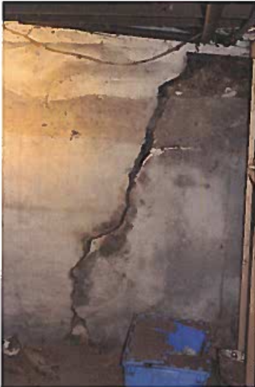
Crack in interior foundation wall
