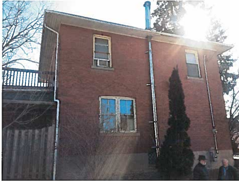
Side elevation- Looking East Note the original w storm windows on the first storey
