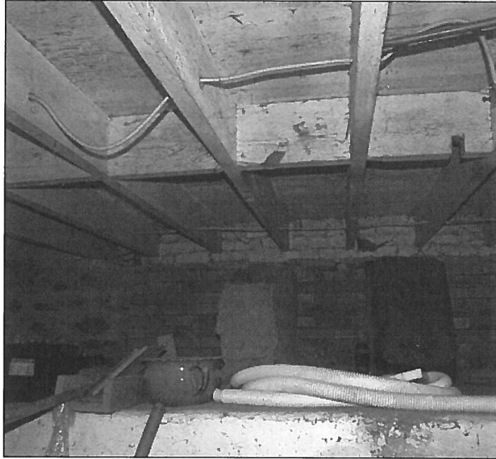
Figure 17: Above: Looking west to brickwork in basement, with rubblestone wall on the left, 2016.
