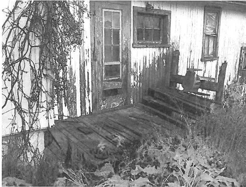
Farmhouse, rotten kitchen walls and porch
