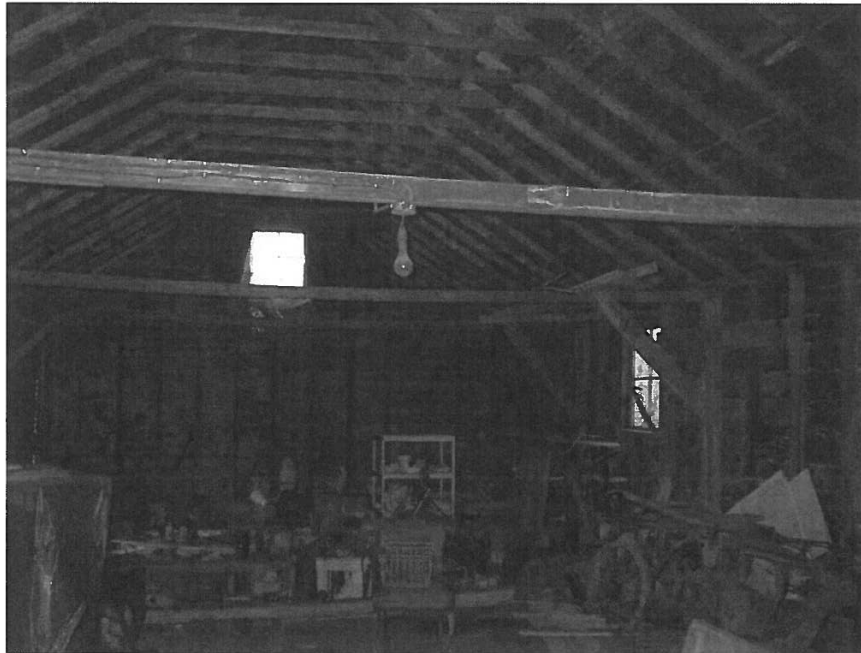
Barn #2, insufficient roof construction
