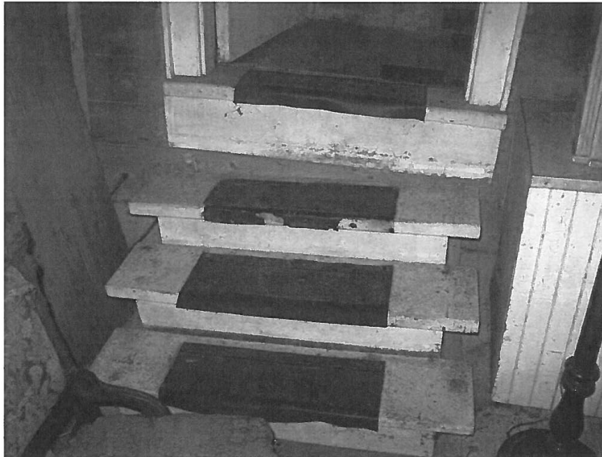
Farmhouse, sagging floors
