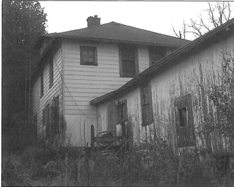
Figure 12: Above: West (rear) façade of main house and north façade of summer kitchen/woodshed, 2016.
