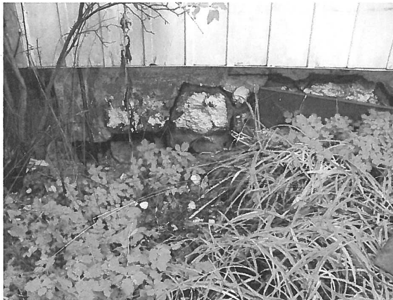
Farmhouse, damaged southwest corner foundations
