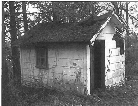
Figure 37: Pumphouse showing a multipaned sash similar to that in the west barn and driveshed, 2016.
