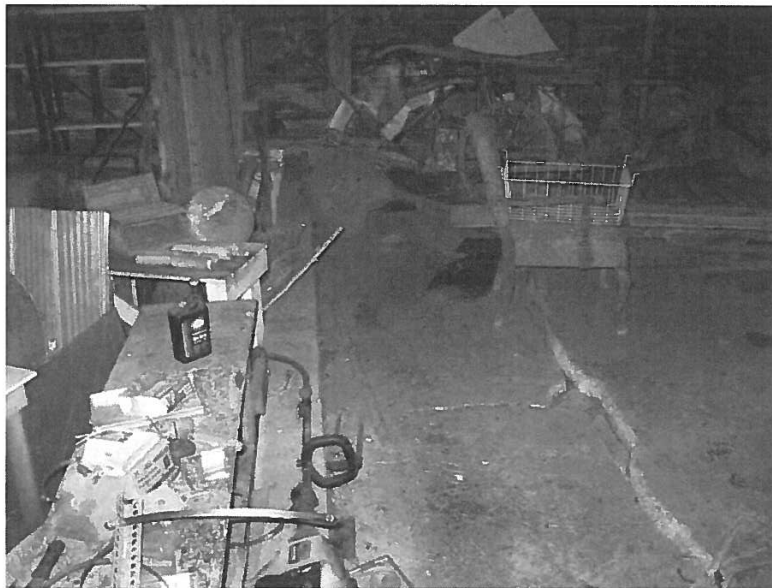
Barn #2, floor slab damage
