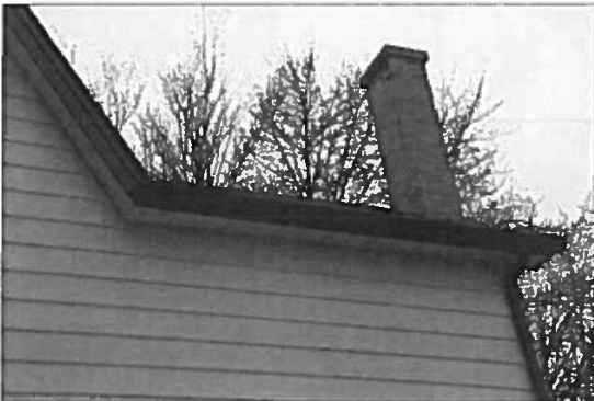
Figure 19 aluminum siding & soffit
