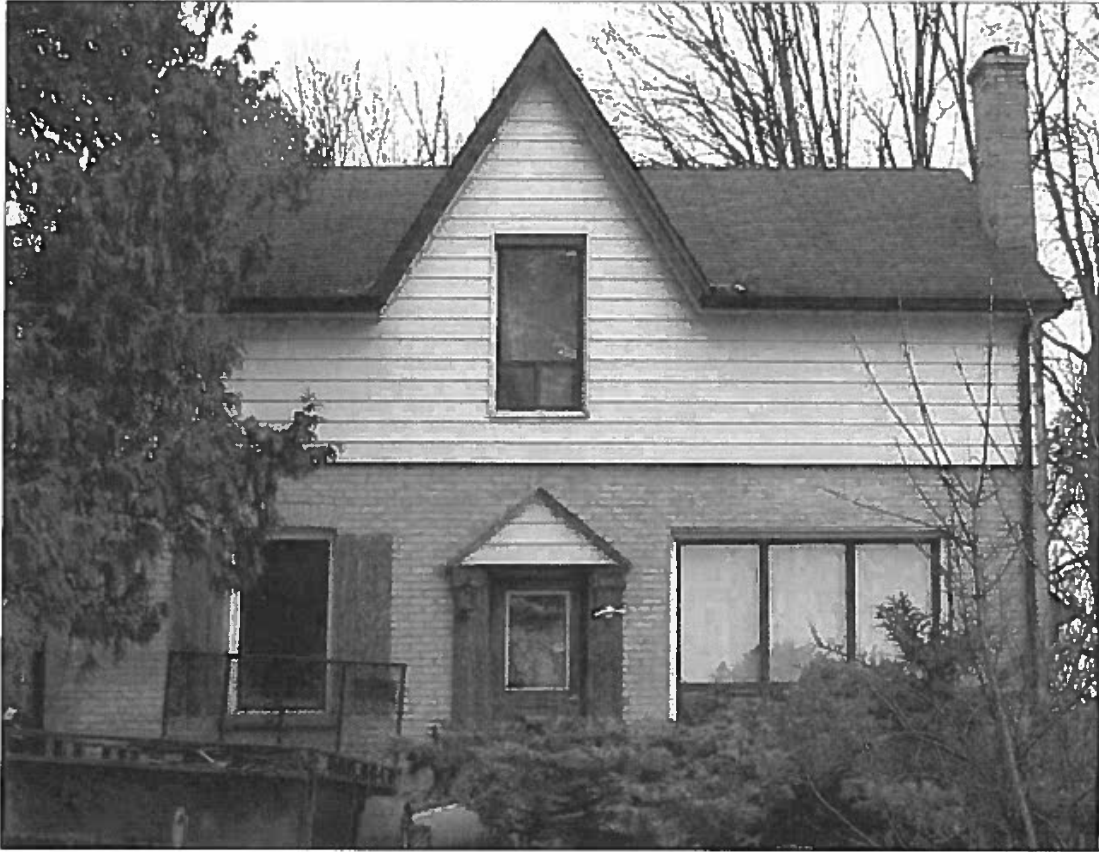
Figure 5 front facade - replacement windows & door, aluminum siding on upper floor & added pediment over door
