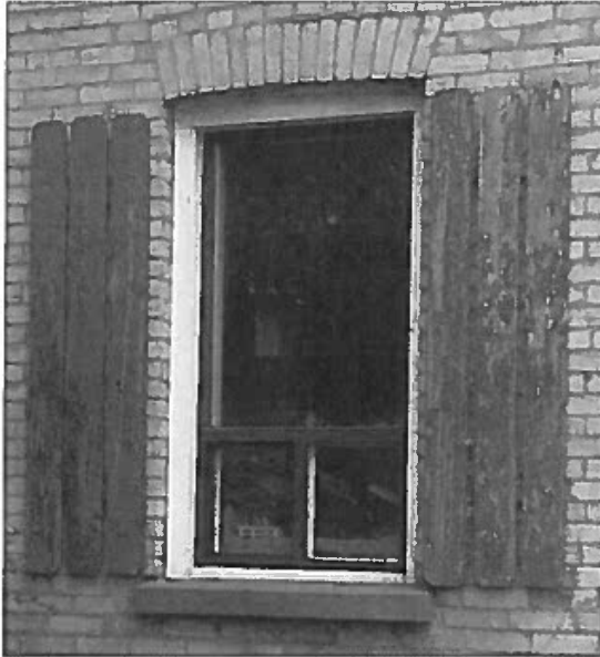
Figure 13 replacement aluminum window, concrete sill, soldier course brick header, non-functional shutters
