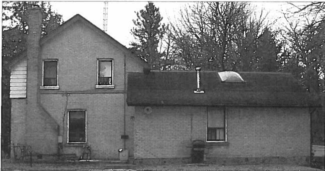
Figure 7 north facade - aluminum siding wraps around corner, new chimney, skylight in summer kitchen wing
