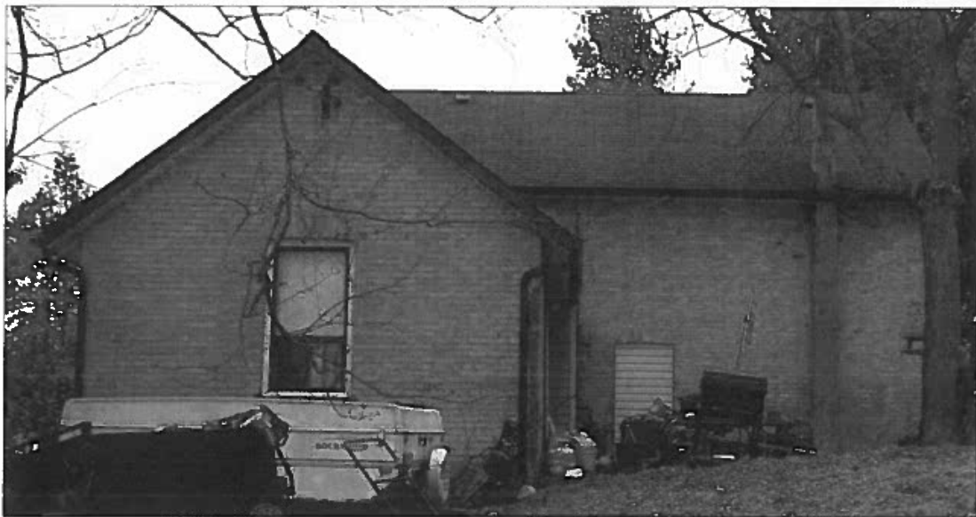
Figure 6 rear (west) facade - rear door blocked, opening sided with aluminum
