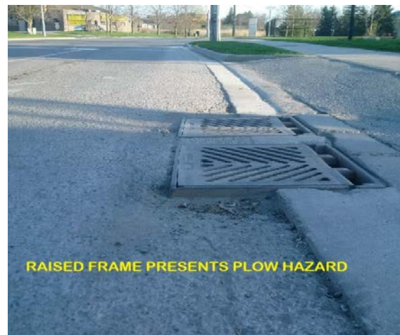
Raised frame presents plow hazard
