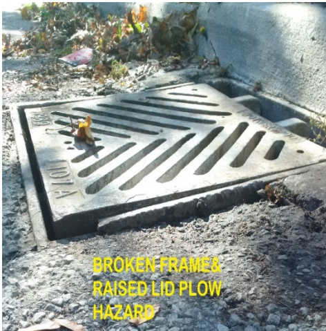
Broken frames raised lid-plow hazard
