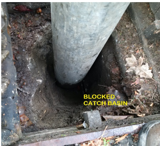
Blocked catch basin
