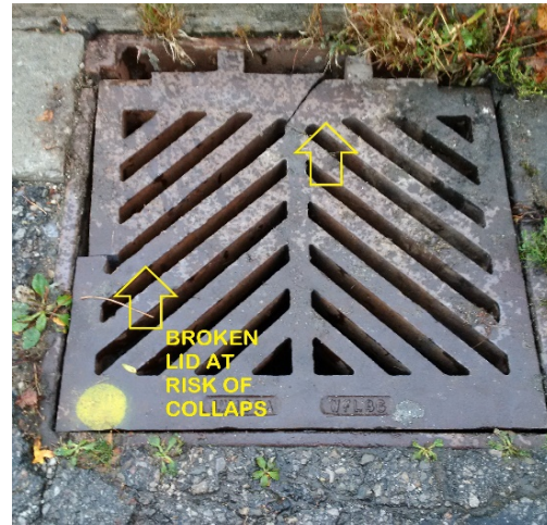
Broken lid at risk of collapse
