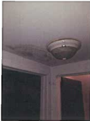
Photo #8 Second Floor Ceiling Elevation (leaks in corridor)
