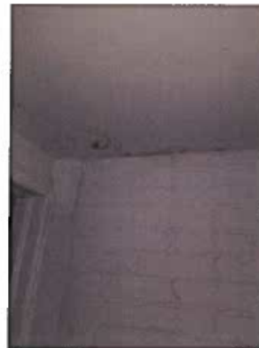
Photo #9 Second Floor Ceiling Elevation (leaks at chimney)
