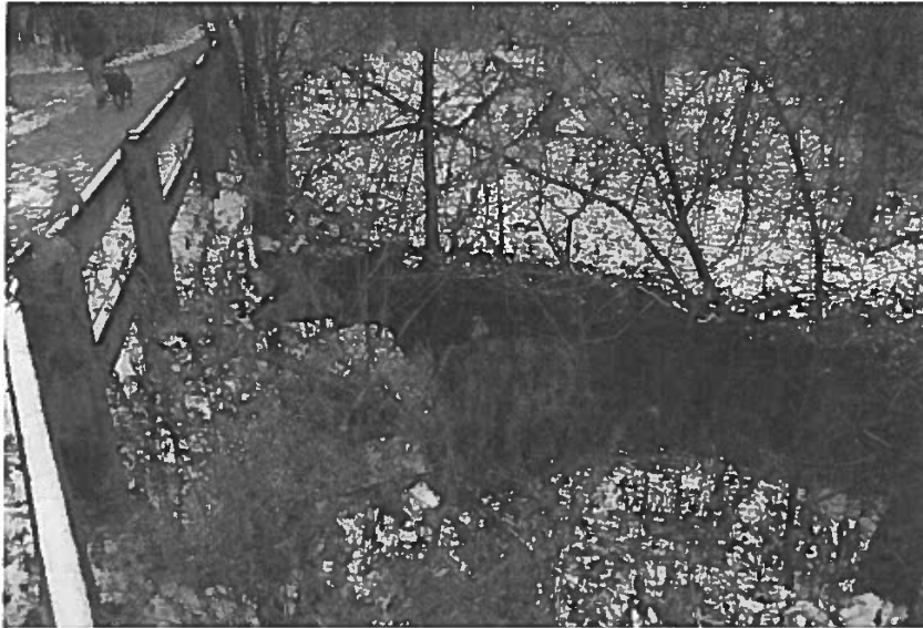
Plate 3: Oblique view of the south side of the subject culvert, looking east.
