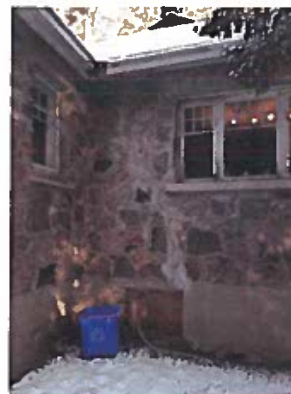
Photo #11 South Elevation (previous repairs; open cracks)
