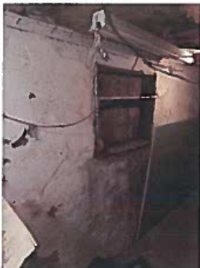
Photo #1: West Foundation Wall (rotted wood/water leakage)
