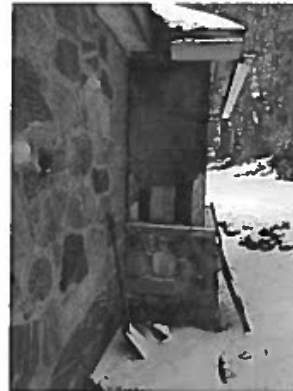
Photo #12 North Elevation (general view; saturated stones at grade elevation; typical)
