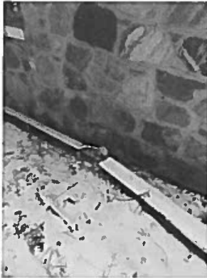
Photo #11 North Elevation (missing stone at grade elevation; typical at several locations)
