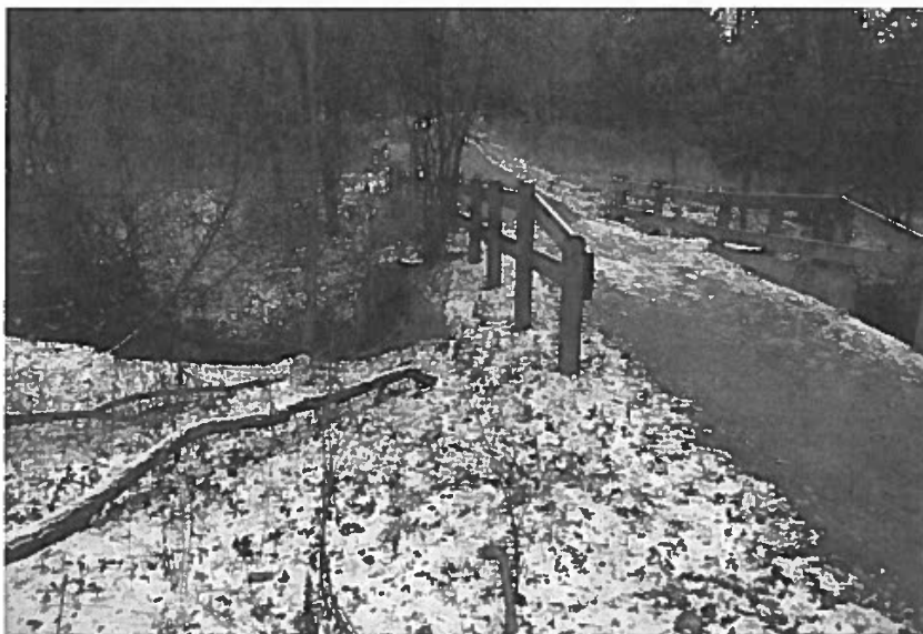
Plate 4: Oblique view of the south side of the subject culvert, looking west.
