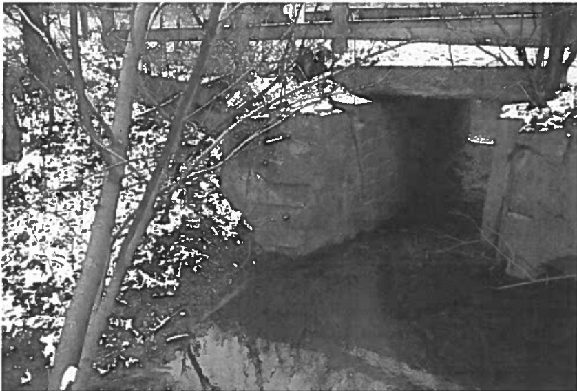
Plate 12: View toward the west wall of the subject culvert. Note the line pattern left by the formwork.
