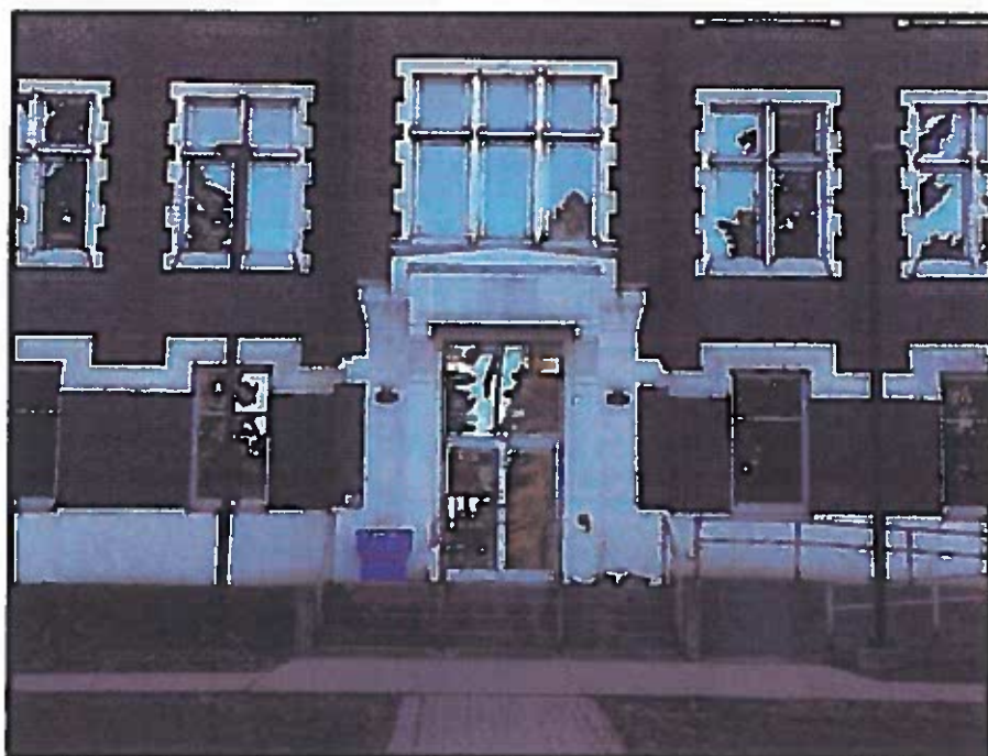
Image 9: Detail of main entryway door of former De La Salle College structure (November 27, 2017; View looking West)
