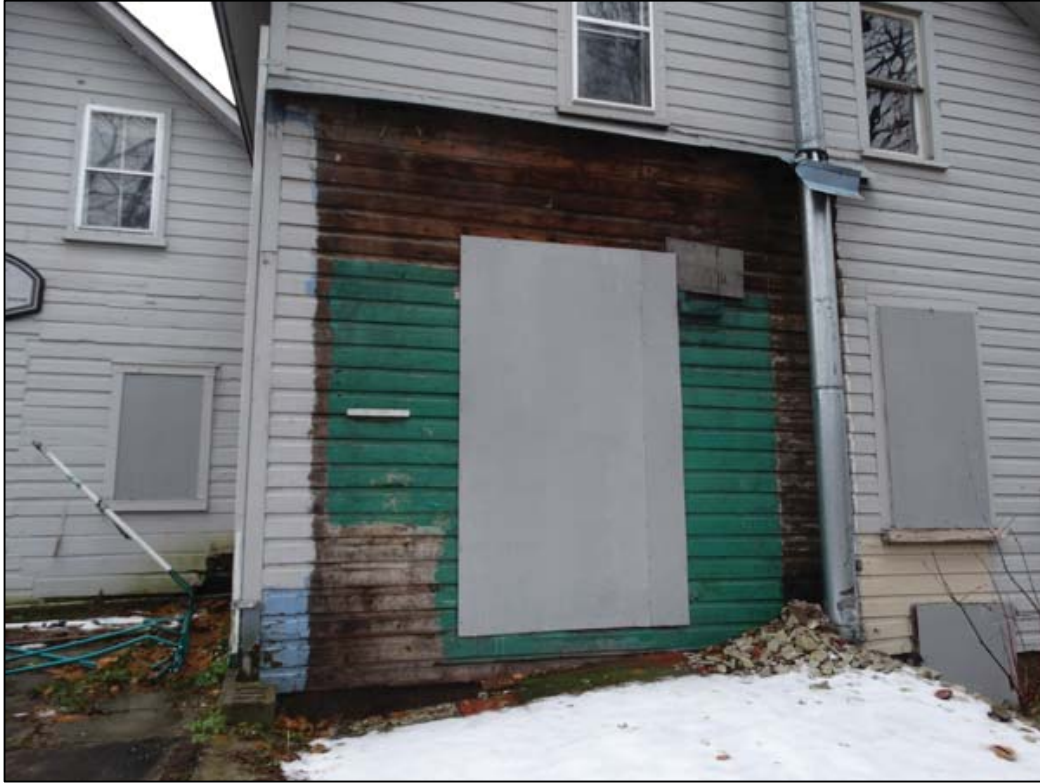
Figure 8: Above: North façade, 2018. Multiple finishes and enclosures indicate this section has been repeatedly altered.
