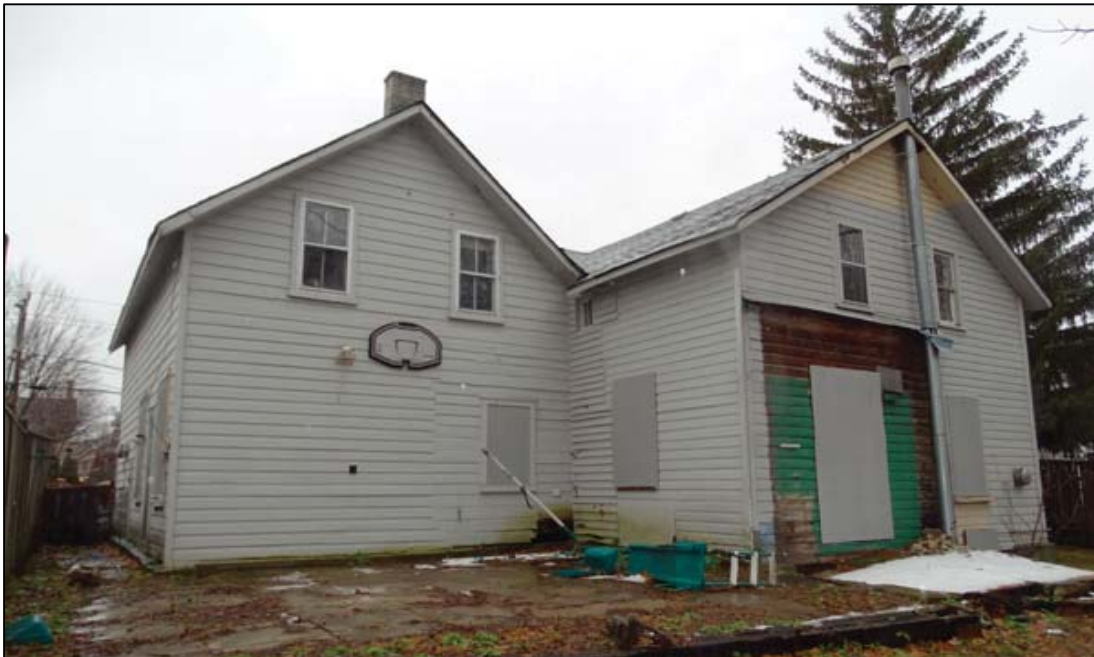
Figure 7: Below: North façade, 2018. The joint where the west and east parts meet is not well aligned. It is possible that a second storey was added to the rear tail of the west part.
