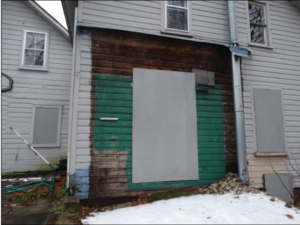
Figure 8: Above: North façade, 2018. Multiple finishes and enclosures indicate this section has been repeatedly altered.
