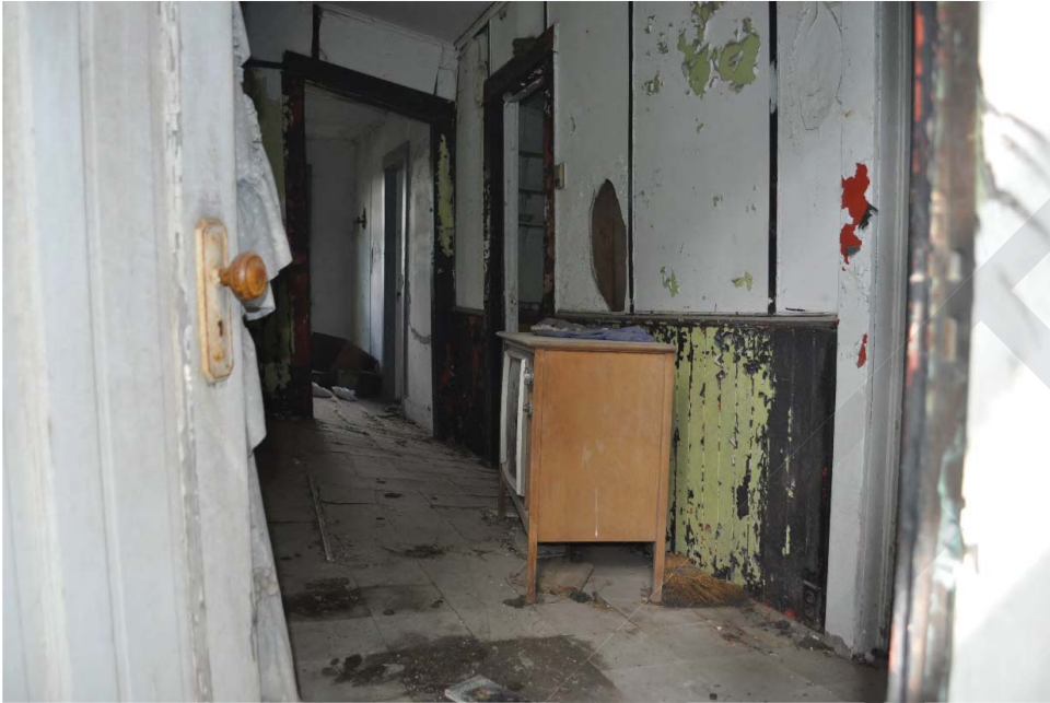
Photo 36: Cottage, interior. Note significant tilt of floor and walls. (CU 2018).
