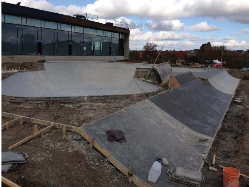
Photo 11 (Looking E, Date Unknown): Skate Park during construction. Photo provided by Town.
