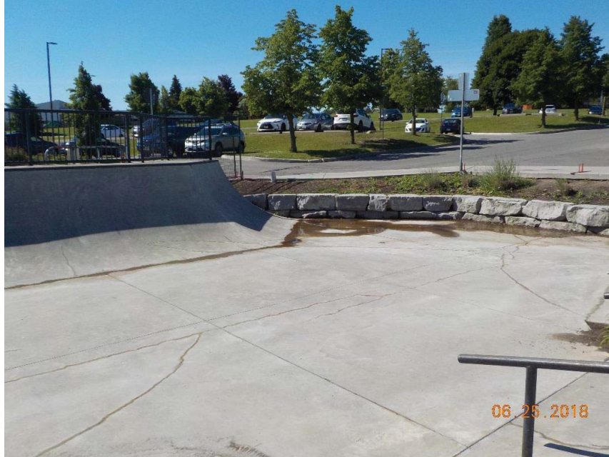
Photo 5 (Looking S): Water ponding observed in the southwest corner of the Skate Park.
