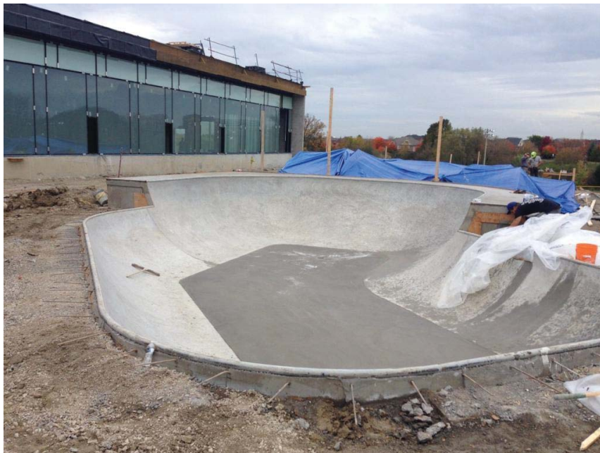
Photo 12 (Looking E, Date Unknown): Skate Park during construction. Photo provided by Town.
