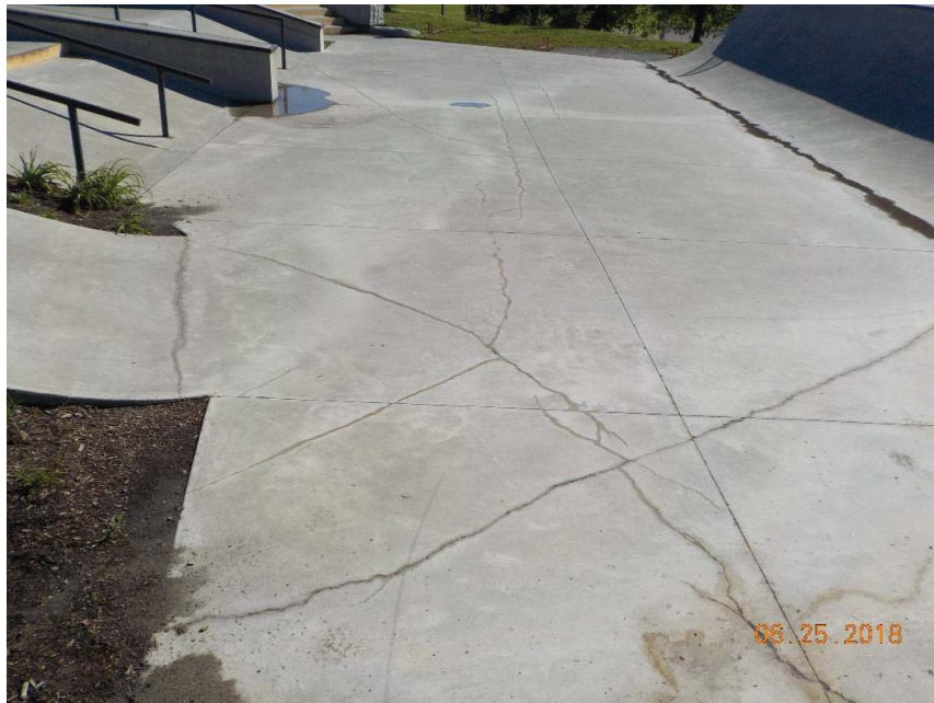
Photo 4 (Looking E): Extensive concrete cracking visible in south section of Skate Park.
