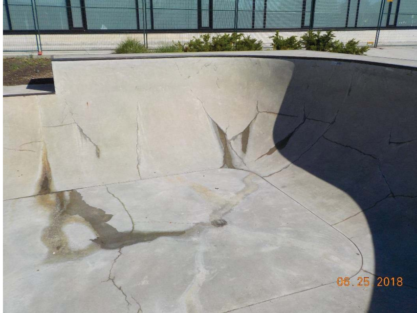
Photo 3 (Looking N): Extensive concrete cracking visible in large bowl.
