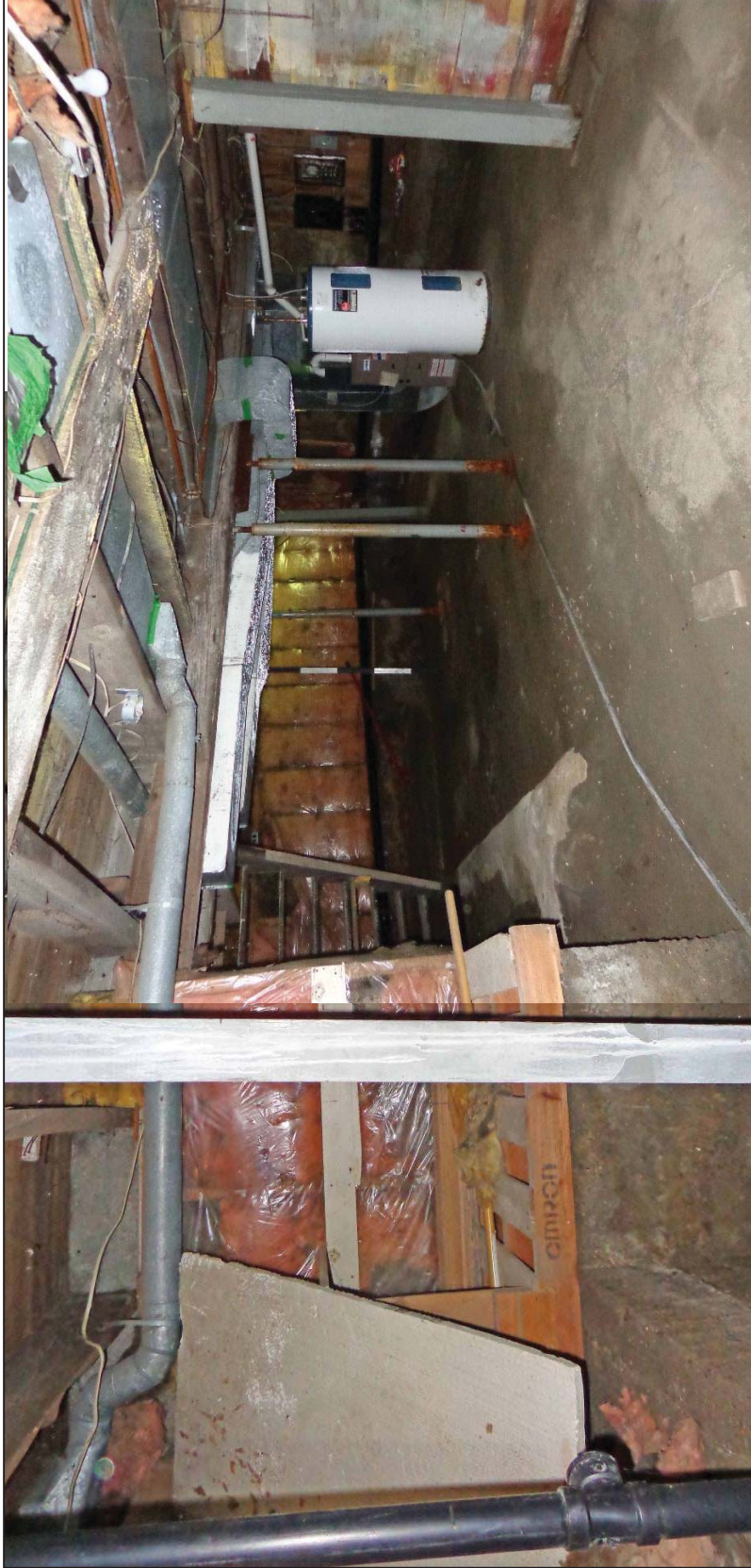
5. View from the southwest corner looking to the north and east walls.
