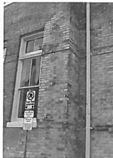
East elevation, showing area of efflorescence (ERA, 2019).
