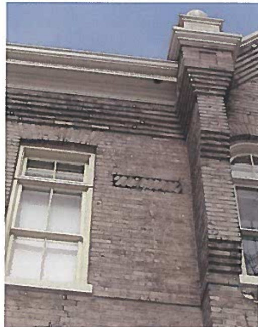
South elevation, detail of wood soffit damage (ERA, 2019).
