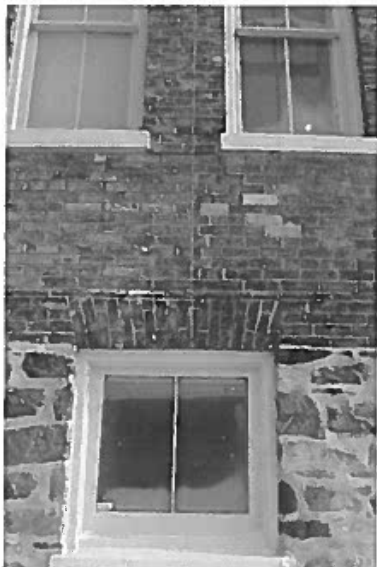
West elevation stone foundation and basement window, showing cracked mortar joints above window (ERA, 2019).
