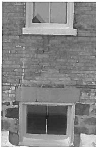
East elevation, showing detail of cracked concrete lintel and cracked and open mortar joints (ERA, 2019).
