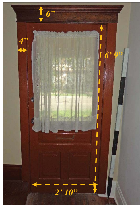
1. Hall – Front Door.
