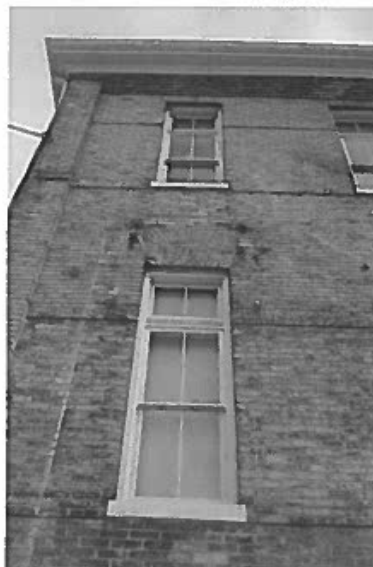
Ghosting on brick from removed fire escape stairs at west elevation (ERA, 2019).
