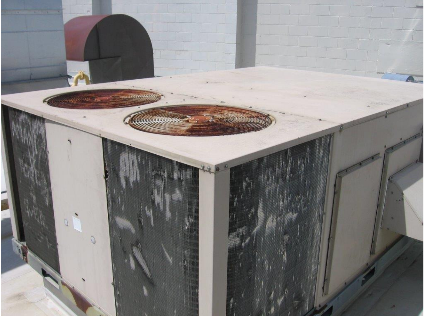
C:\Users\Karen Oretol\Pictures\72132 - 2016\ACC rooftop hvac condensers 001.jpg
