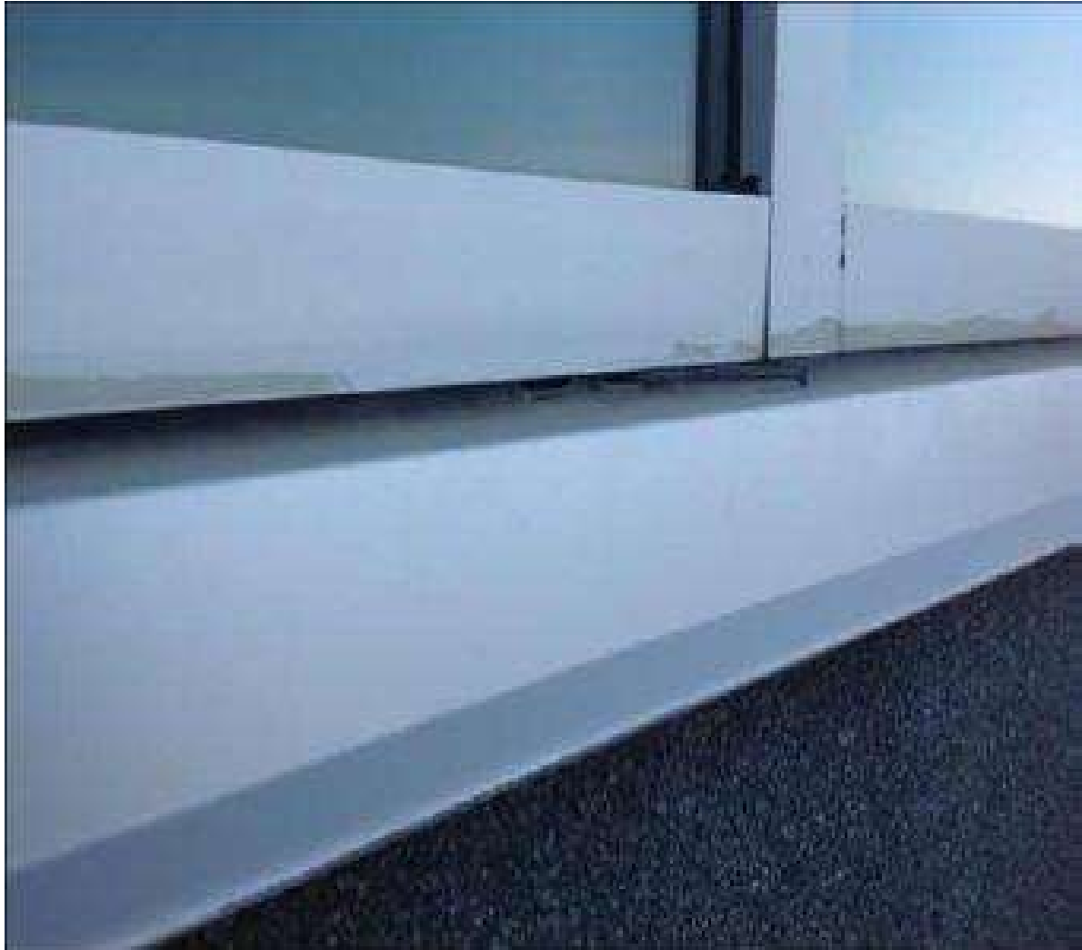
Deteriorated Sealant West Windows
