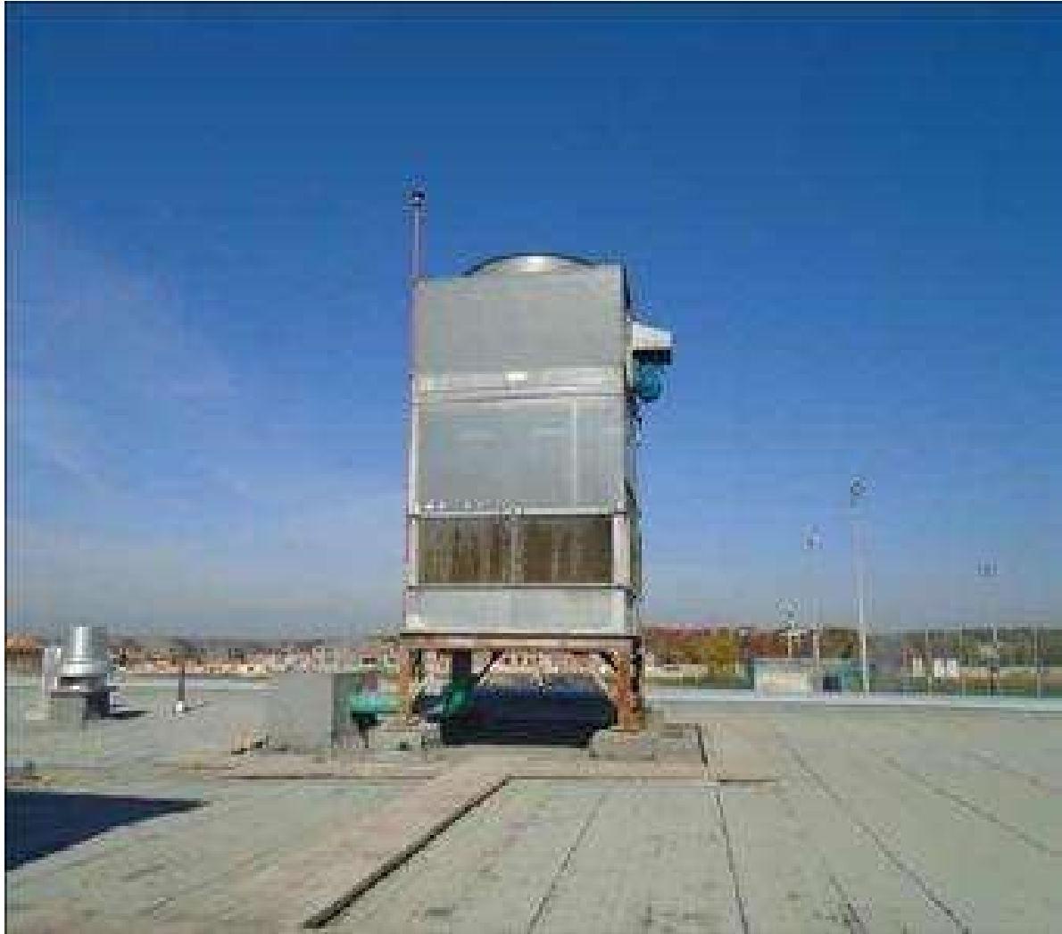
Cooling Tower installed in 2005
