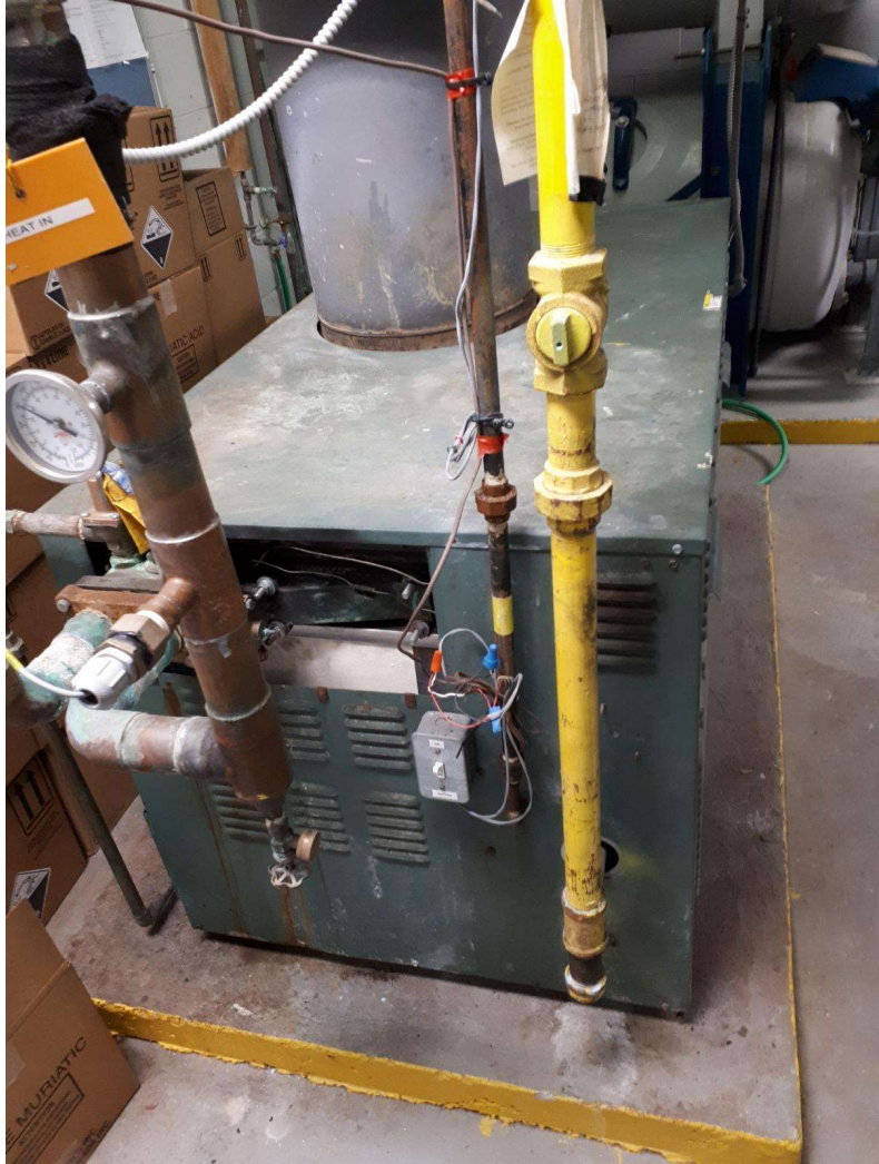
Pool Boiler 2.jpeg
